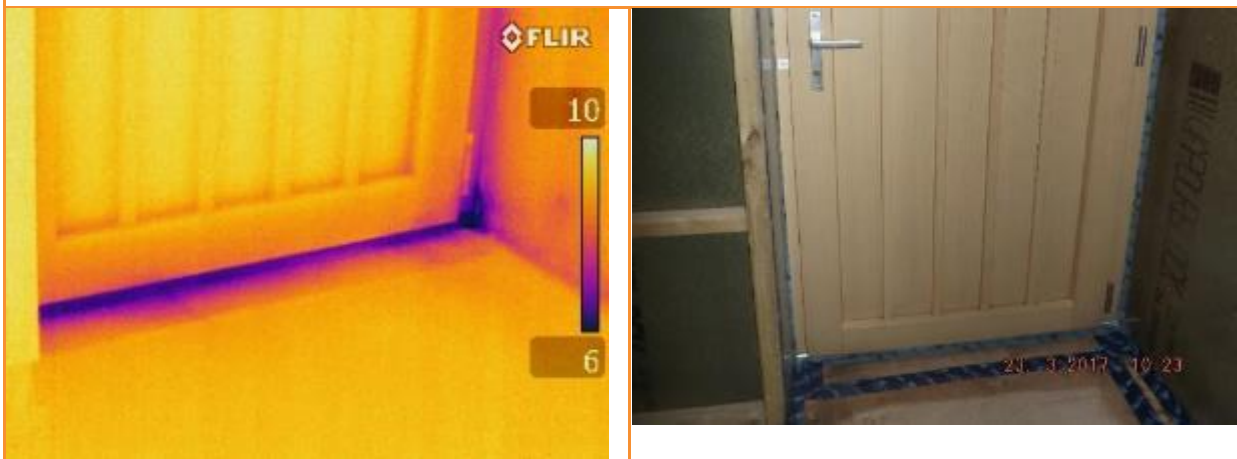
5.04: Internal thermographic image whilst house is depressurised showing leakage across base of internal door to garage, particularly at corner.
