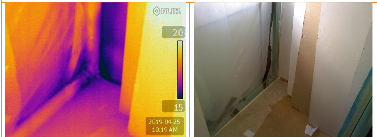
5.08: Thermographic image showing substantial leakage at the bottom corner and side of the existing rear door, which has yet to be replaced
