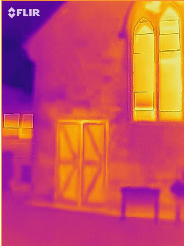
5.16: External thermographic image while building is pressurised showing leakage of warm air (yellow) at side and top of fire escape doorway from main hall
