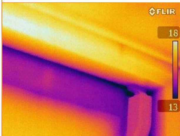
5.37: Thermographic image of major leakage across top of side door whilst depressurising
