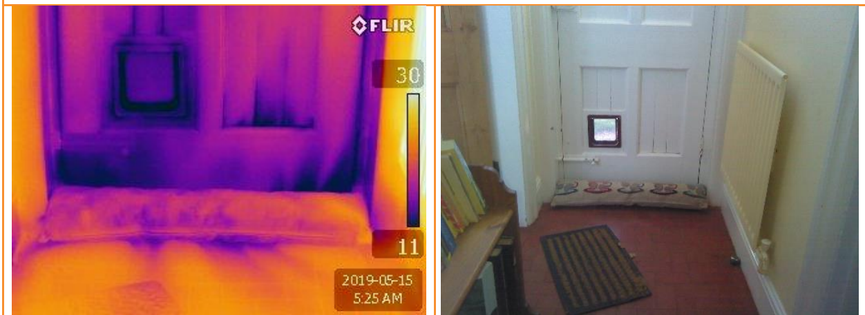
5.07: Internal thermographic image whilst house depressurised, showing substantial leakage on base of side door, also around cat flap, through the panels of the door and beneath the threshold
