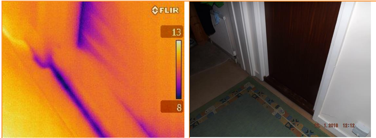
5.45: Thermographic image showing substantial leakage at lower side and beneath threshold
