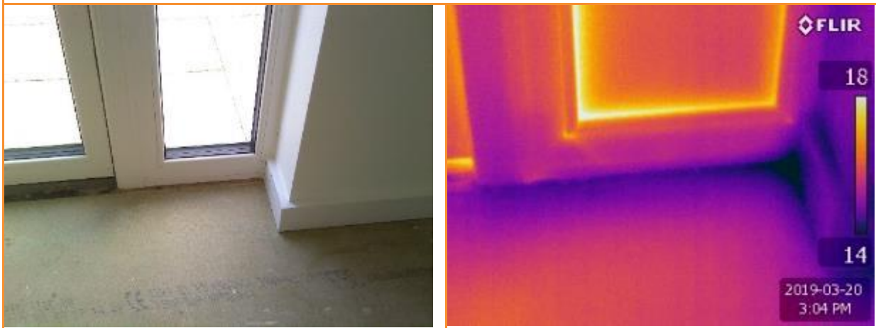
4.6: Internal thermographic image whilst house is depressurised showing leakage at base and right side of rear door.
