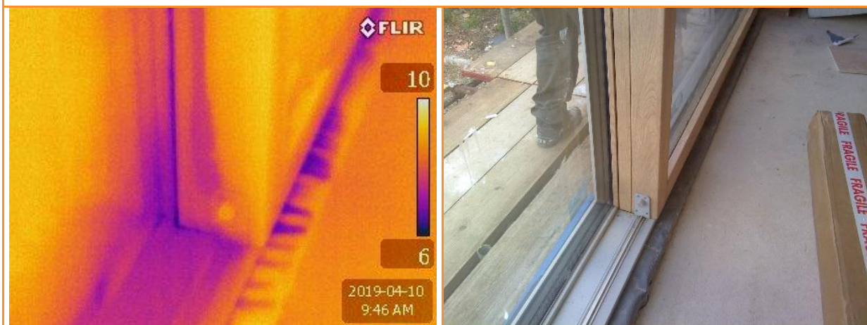
4.16: Thermographic image showing numerous leakage locations beneath the threshold of the first set of large sliding doors, also along the vertical meeting rail, particularly at its base
