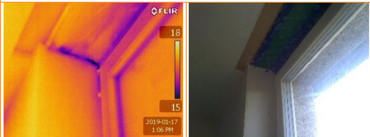
4.4: Internal thermographic image whilst house is depressurised showing leakage at top of large sliding doors.
