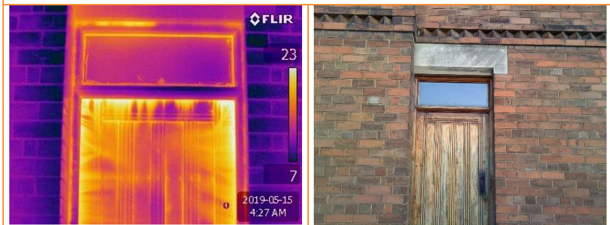
4.12: External thermographic image whilst house pressurised showing leakage around the side door, both at the top and sides of the door, but also across the top of the glazed panel above the door
