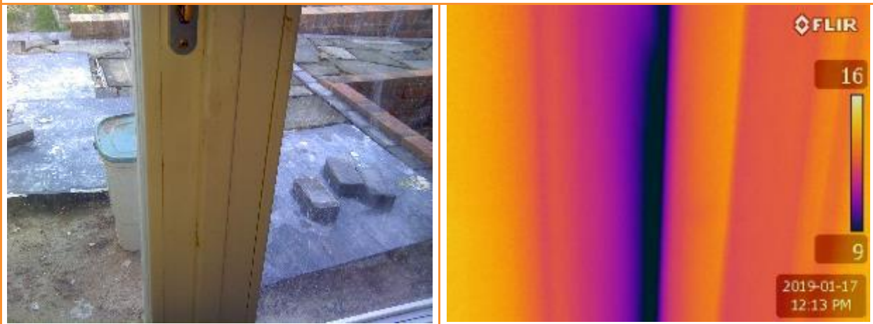
4.3: Internal thermographic image whilst house is depressurised showing leakage on meeting rail of French windows where draughtseals are ineffective.
