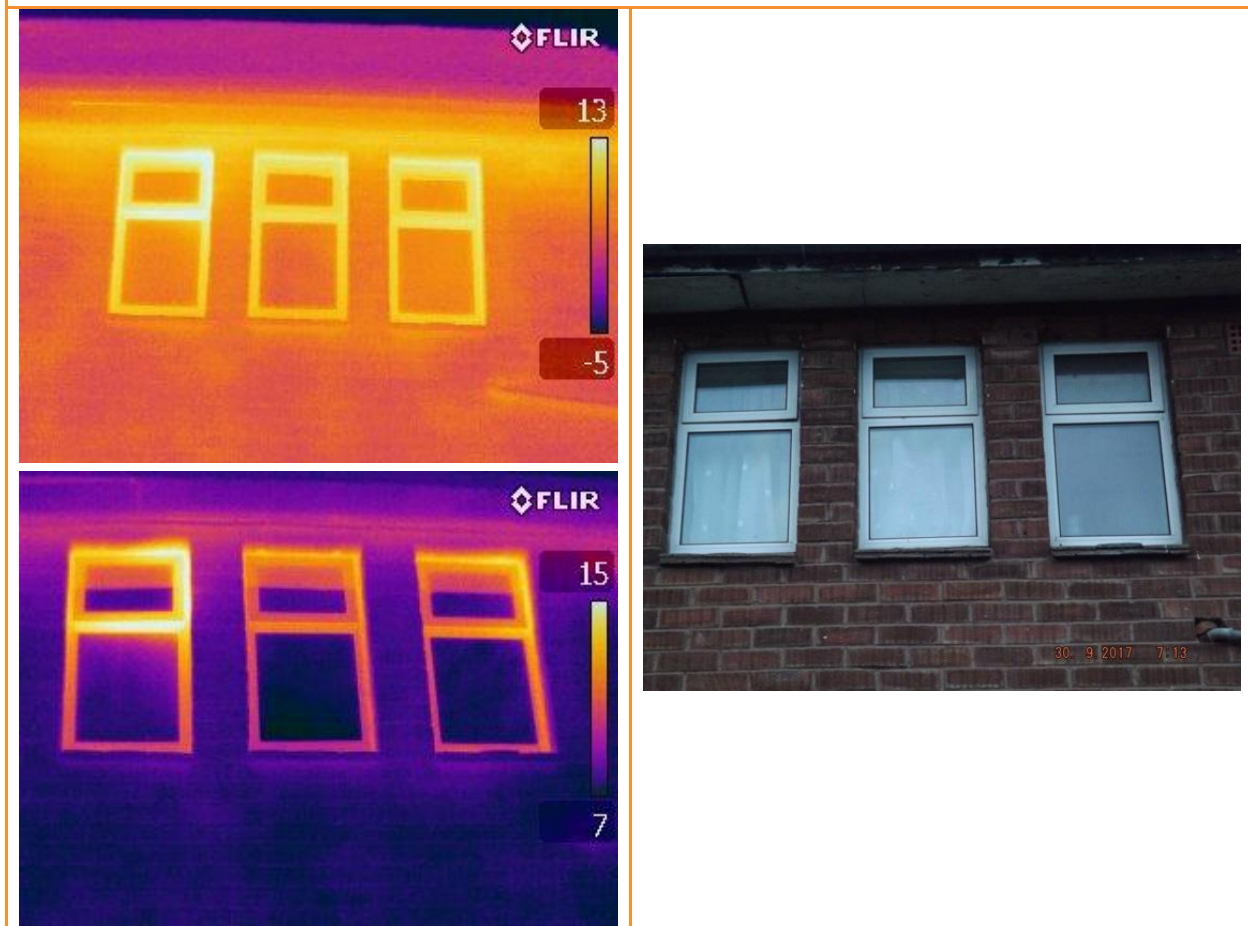
3.17: Thermographic image of stairs and WC windows, first floor, before pressure differential applied (top) and after pressure differential applied (bottom)
