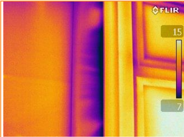
2.45: Thermographic image of major leakage at side of window frame whilst depressurising
