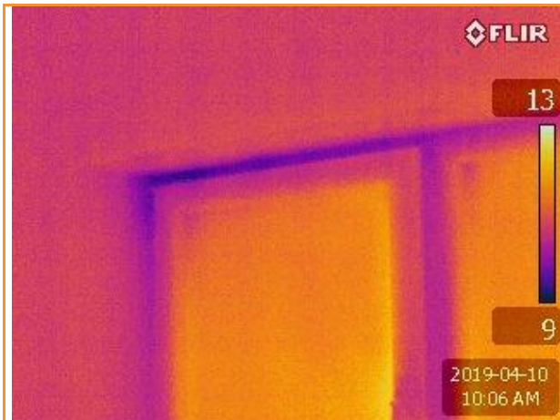
2.36: Thermographic image showing leakage at head of first floor window
