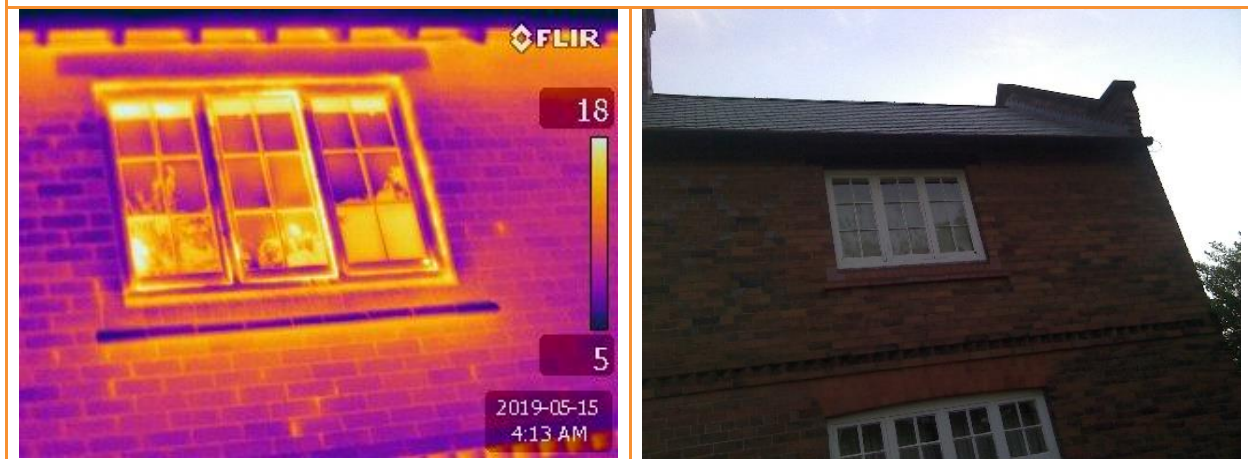
2.19: External thermographic image whilst house pressurised, showing leakage around upper right front window. Also, eaves leakage and leakage under brick detail visible
