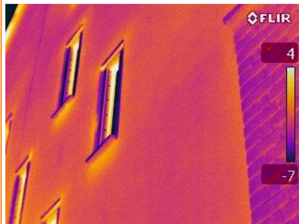
2.49: Thermographic images of window sills at east end of building before pressure applied (top), then after pressure applied, showing noticeably more heat loss (bottom)
