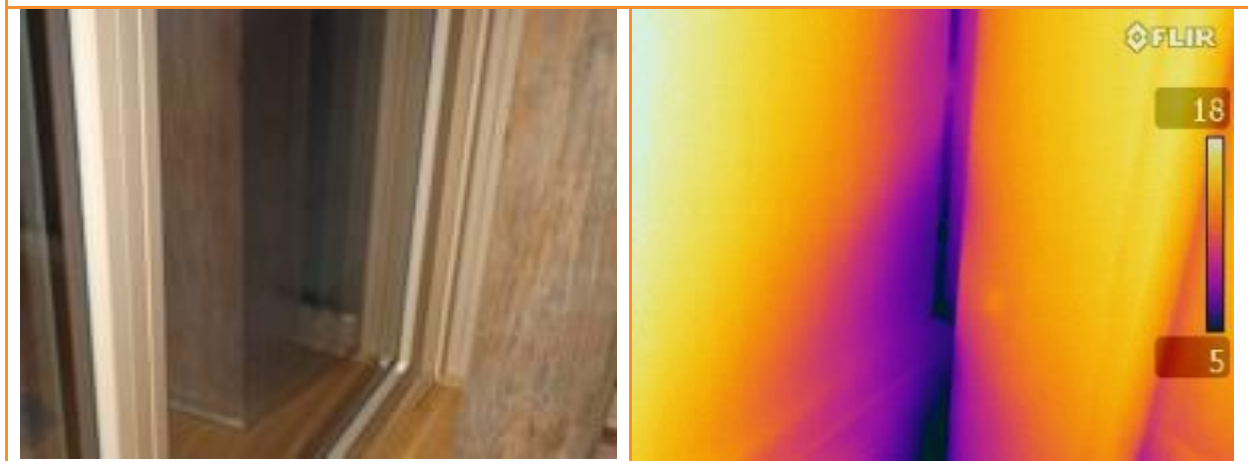
2.09: Internal thermographic image whilst dwelling is depressurised showing leakage down the side of a window frame.
