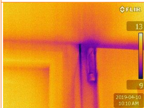
2.38: Thermographic image showing leakage between sections of window just below the head, first floor bedroom, also around hinge
