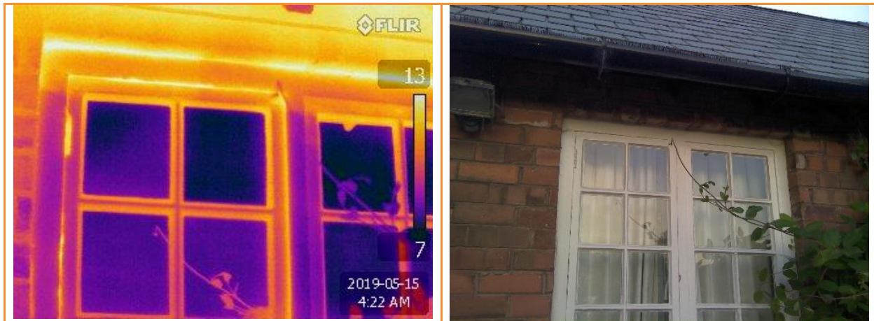
2.17: External thermographic image whilst house pressurised showing leakage around the opening window but also between the window frame and the wall above
