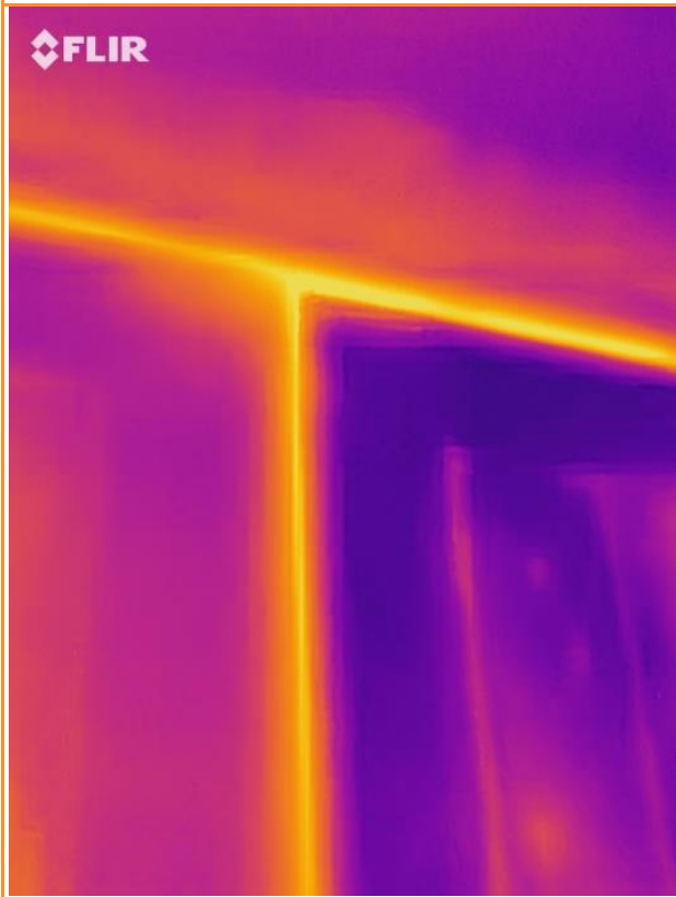
2.29: External thermographic image while building is pressurised showing leakage of warm air (yellow) at side and top of window in gents' toilet.
