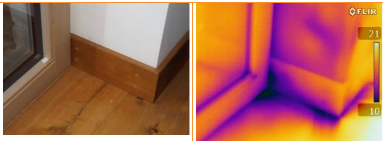
2.07: Internal thermographic image whilst dwelling is depressurised showing leakage at lower corner of opening.
