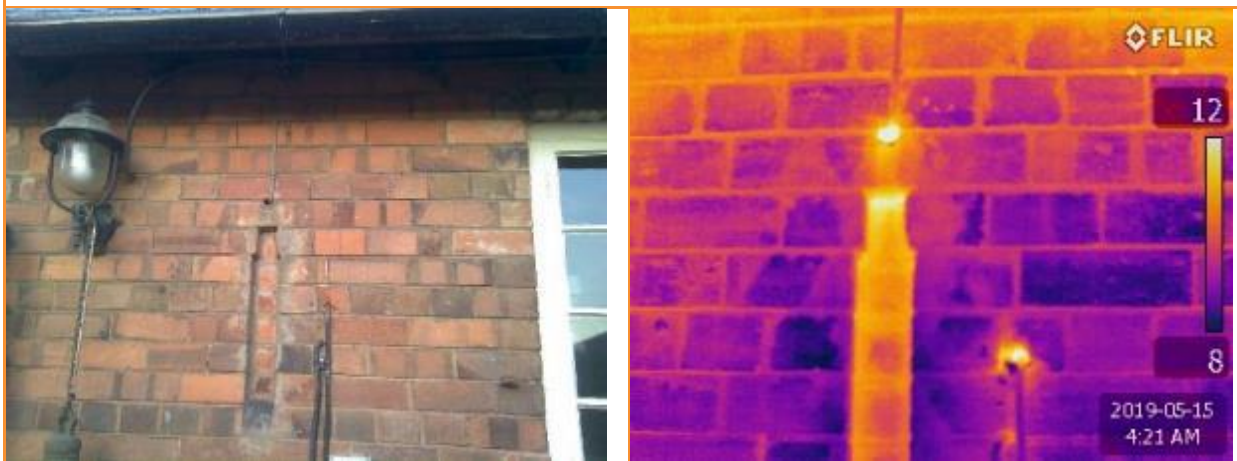
12.04: External thermographic image whilst house is pressurised showing leakage at top of brick alcove.
