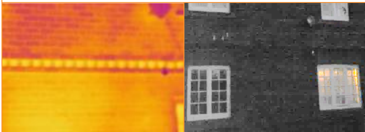
1.07: External thermographic image whilst house pressurised, showing significant heat loss from the decorative feature along the external edge of the intermediate floor
