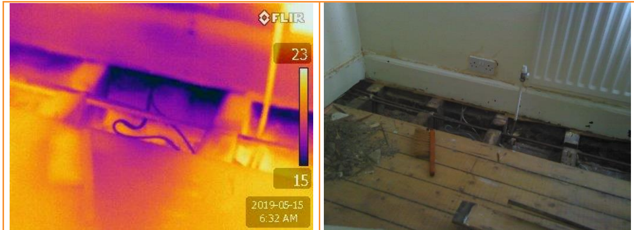
1.05: Internal thermographic image with house depressurised, showing substantial leakage around perimeter of intermediate floor where floorboards lifted in bedroom to side of house
