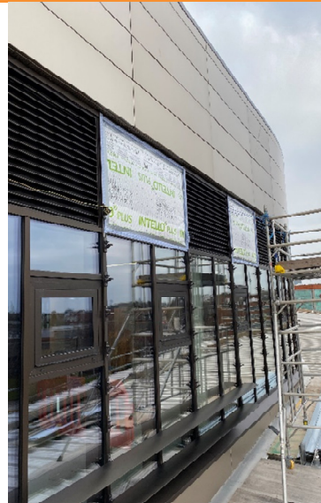
A1.4) External view of temporary sealing over ventilation grilles from L2 roof
