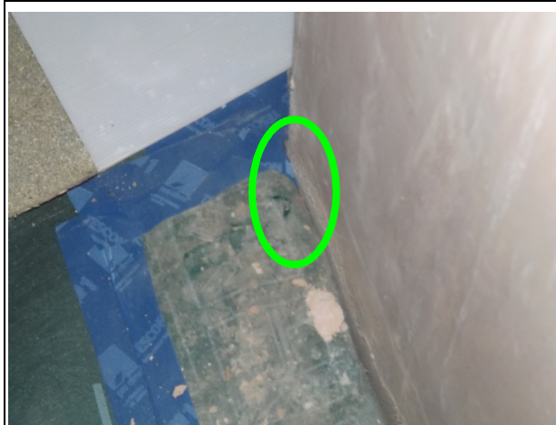
P12) Damage to subfloor membrane identified & then repaired before Vacupor insulation and floating floor installed (item 6)
