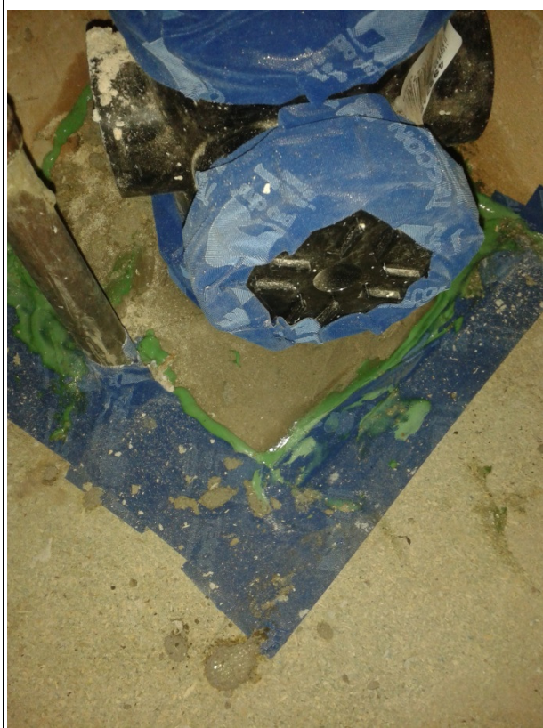
P8) Partially effective sealing at base of soil vent pipe, also tape seal over joints (item 3)
