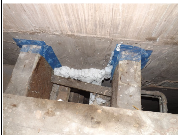
P16) Tape and some foam sealing around floor joists into party wall (item 10)
