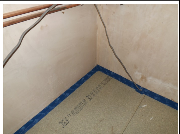
P13) Edge of floating floor sealing with Tescon tape to eliminate edge leakage (item 6)
