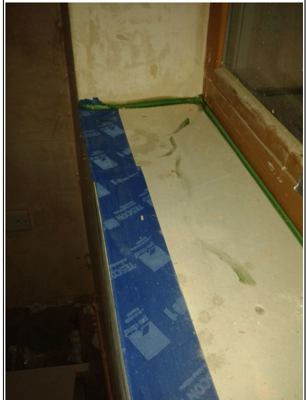
P9) Tape along front edge of window sill to stop leakage at corner joint in plasterboard (item 8)
