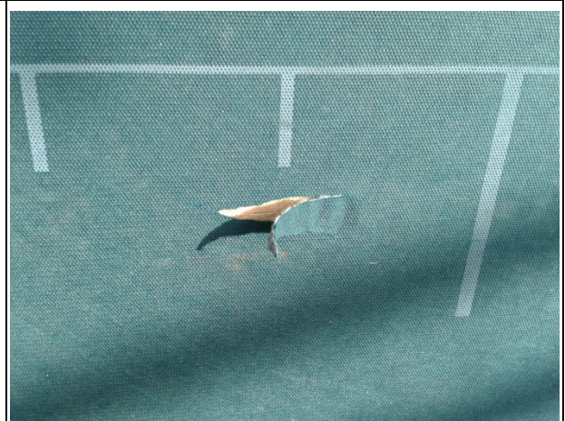
P17) Torn DA membrane, viewed externally (item 13)
