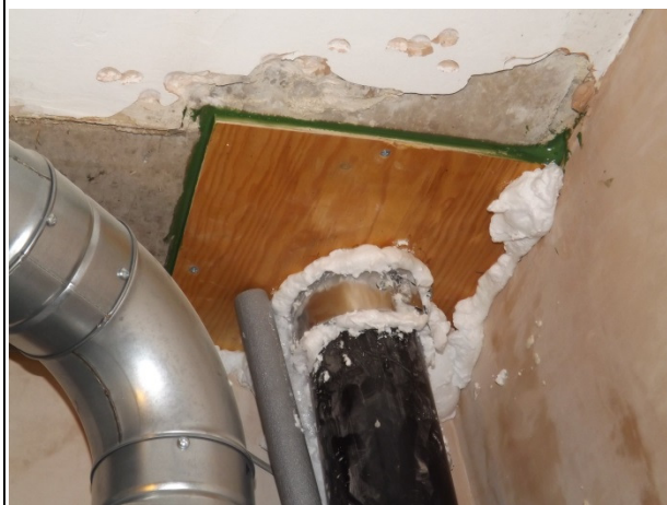
P10) The timber battress at the top of the soil vent pipe in both No's 3 (shown) & 18 has had to be resealed more than once (item 4)
