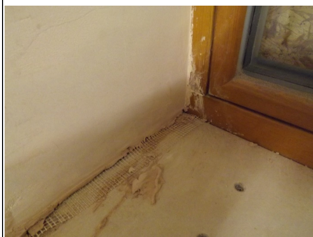
P14) Leakage along unfinished edge of window reveal (item 8)
