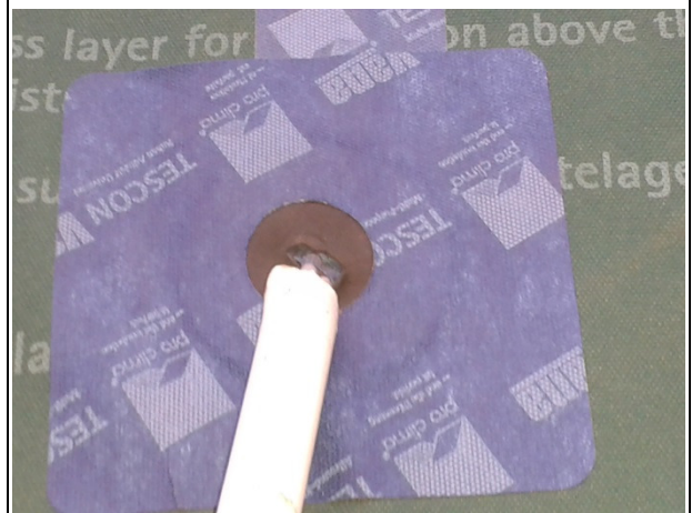
P11) Ineffective seal where cable penetrates front façade (item 5)
