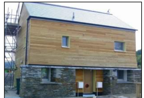
Final acceptance test, July 2010 Passivhaus certification test Worsened to 0.23 AC/hr @ 50 Pa – damage to floor membrane
