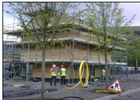
Post 1st-fix test, May 2010 After wall penetrations sealed Improved to 0.20 AC/hr @ 50 Pa
